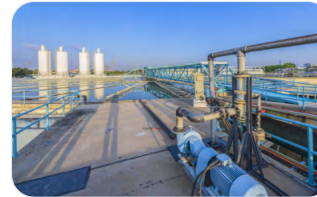
Wastewater System Monitoring
